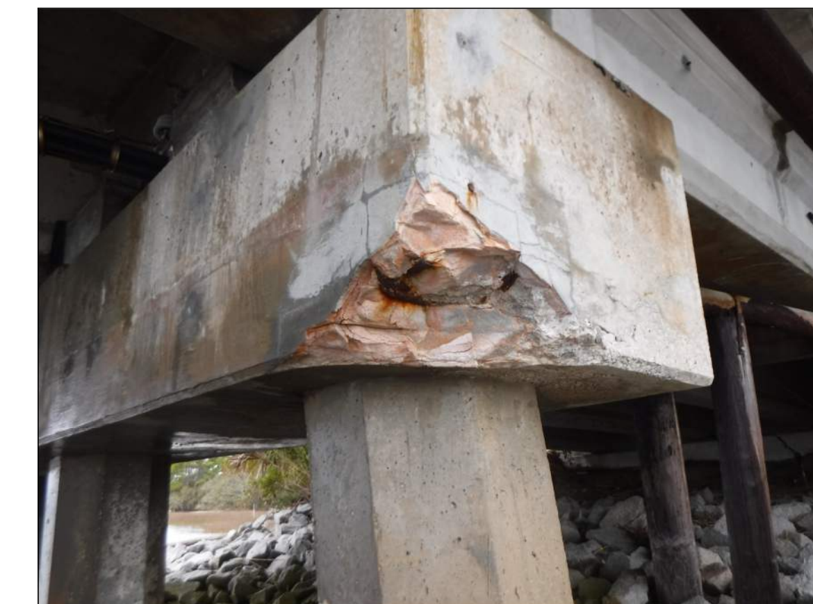
PHOTO 2: TYPICAL SPALL REPAIR ITEM
