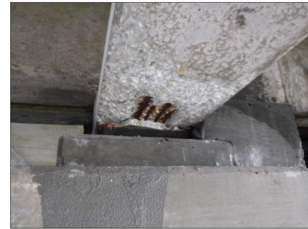
PHOTO 1: TYPICAL SPALL REPAIR ITEM
