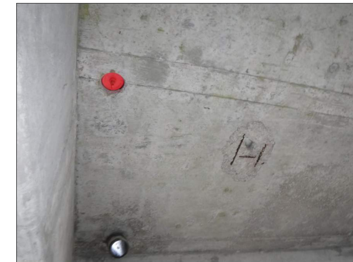
PHOTO 1: TYPICAL SPALL REPAIR ITEM
