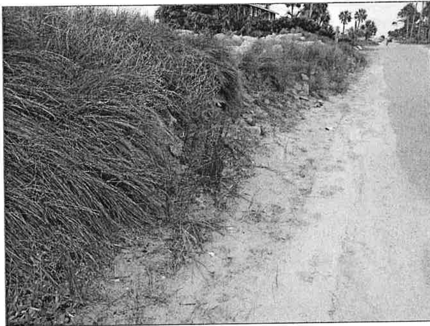
Photograph 3: Minor erosion of the backslope adjacent to Porpoise Drive, near Sta. 13+50
