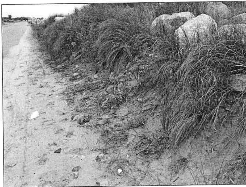
Photograph 4: Minor erosion of the backslope adjacent to Porpoise Drive, near Sta. 13+50
