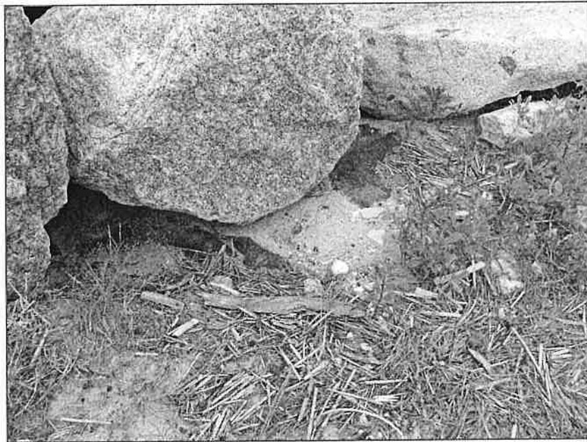
Photograph 2: Exposed filter fabric near Sta. 10+00
