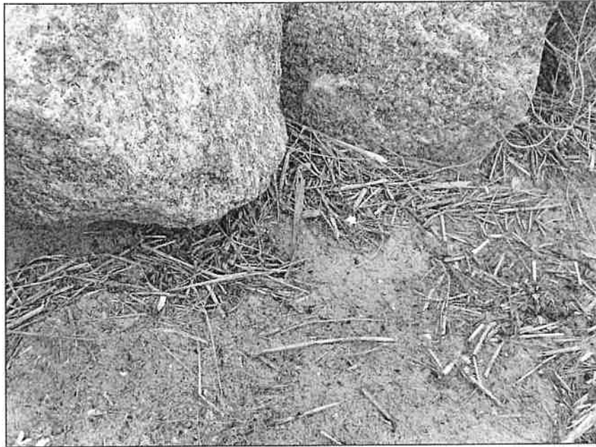
Photograph 1: Water coming through revetment near Sta. 10+00
