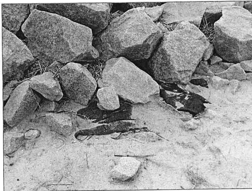
Photograph 6: Exposed filter fabric and water coming through the revetment, near Sta. 19+50
