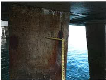
Photo #: 13 Caption: P13-G South, All faces, Vertical cracks [up to 36"L x 1/16"W with RS]
