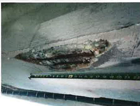
Photo #: 7 Caption: BM25-3, [8.3'] from BRG25-3(A), failed patch [up to 18"L x 6"W x 1"D] with [3] exposed PS strands [up to 90% SL]
