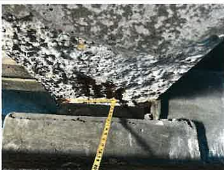
Photo #: 5 Caption: BM7-3 at BT8, bottom flange, spall [up to 36"L x 18"W x 2"D] with [4] exposed PS strands [up to 100% SL]
