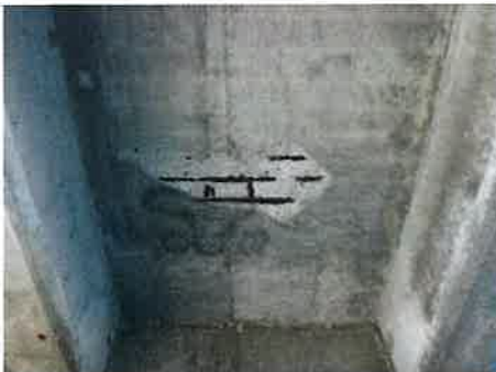
Photo #: 3 Caption: Underside of deck, Span 2, Bay 1, spall [2'L x 5"W x 2"D] with [3] exposed transverse and [2] exposed longitudinal reinforcing [1/8" SL]
