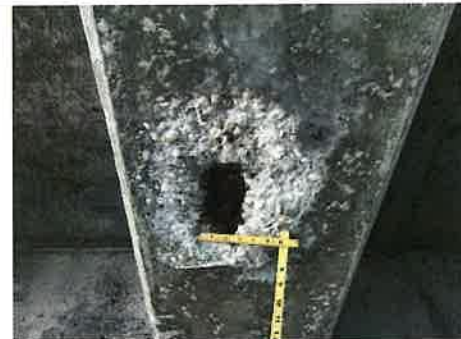
Photo #: 4 Caption: BM6-2, [32"] from BRG6-2(B), spall [15"L x 12"W x 1"D] with [2] exposed strands [50% SL]
