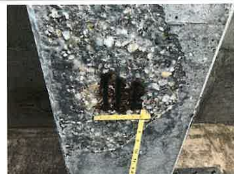
Photo #: 6 Caption: BM7-2, [2.3'] North of BRG7-2(A), bottom flange, spall [22"L x 14"W x 2"D] with [3] exposed PS strands [up to 50% SL]
