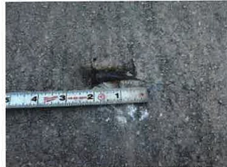
Photo #: 2 Caption: SN37, Southbound lane, near midspan, rebar protruding from deck [up to 1/4"H x 2"W] worn smooth by traffic. Recommend grinding flush to deck
