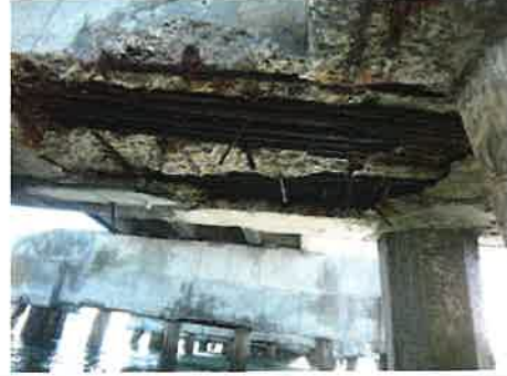
Photo #: 10 Caption: BT13, underside of Retrofit Cap, spalls [up to FW x up to FL x 1'H] with ERB [up to 100% SL]
