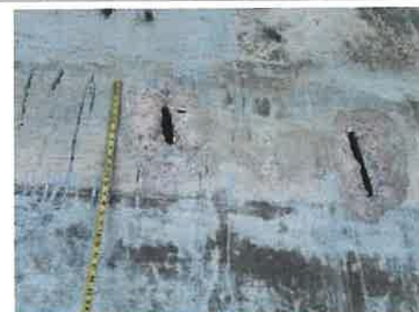
Photo #: 8 Caption: BT13, lower retrofit cap, [3'] above bottom of cap, above Pile E, [2] spalls [up to 10"L x 16"H x 1.5"D] with ERB [1/8" SL]
