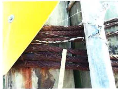
Photo #: 14 Caption: Southwest Dolphin, steel cable wraps, corrosion [up to 5% of strands, 100% SL]
