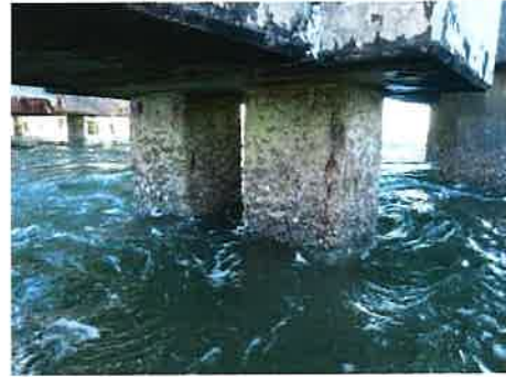
Photo #: 12 Caption: P9-B South, SW Corner, Vertical crack [20"L x 1/16"W with RS]
