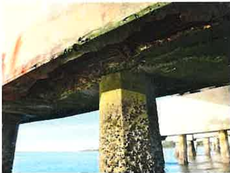
Photo #: 11 Caption: BT10, underside of Retrofit Cap, spalls [up to FW x up to FL x 1'H] with ERB [up to 100% SL]
